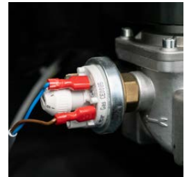
Gas inlet low pressure switch
